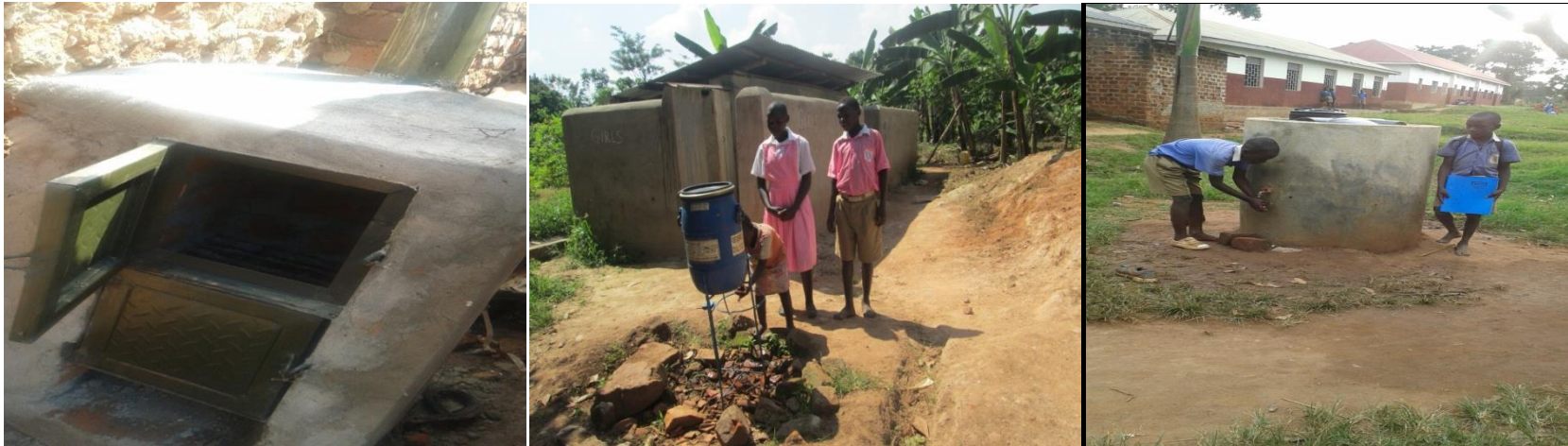
The photos above show an incinerator constructed at Seeta UMEA p/s, the newly constructed latrine at Sitankya p/s and a hand washing facility put up at Kyabakadde R/C p/s respectively.
